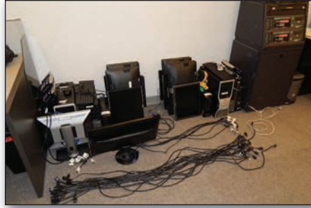
Computers and cabling.
