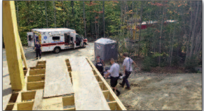
9-16-17 – 35 Ambulance 2, Rescue 1, Utility 1 working a construction site accident. Technical Rescue required to carry out patient.
