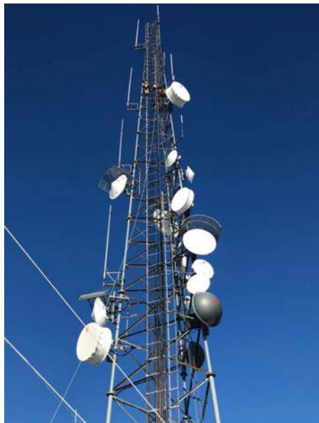
Figure 3: Blue Job Mountain Antennas
