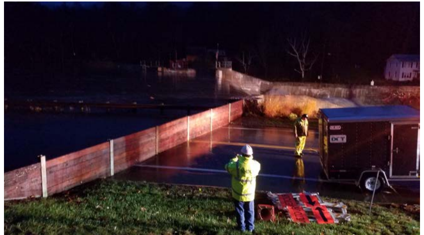
Figure 8: Campton Pond Dam Flooding - October 2017
