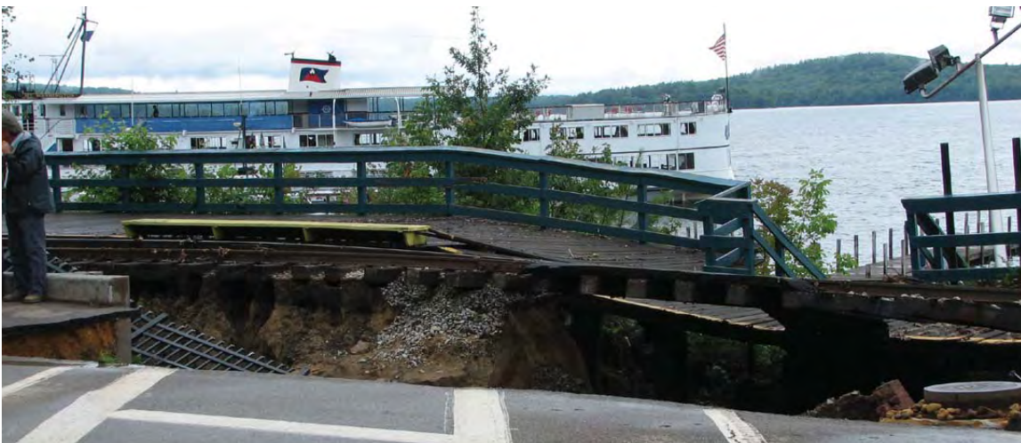
The Boardwalk and railroad tracks at Weirs Beach sustained heavy damage in August.
