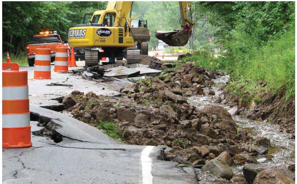
NH Route 106 washed out August 7 after torrential rain hit the area.
